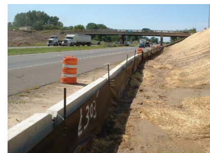
Figure 20. Silt fence protecting a highway and underground fiber optics cable.
