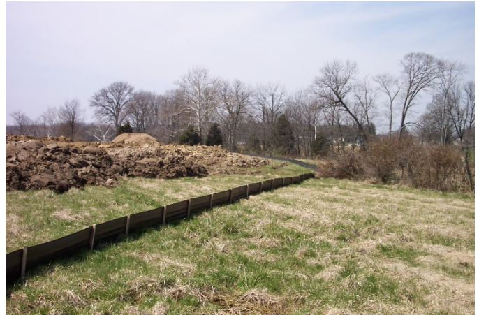
Figure 1. A silt fence at the perimeter of a construction site. Photo Credit: USEPA/Wikimedia
