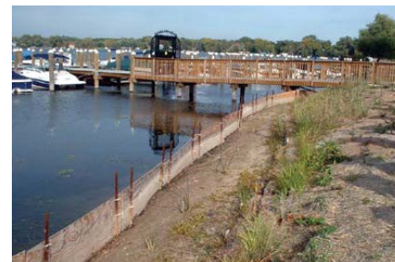
Figure 21. Silt fence protecting a lake shore.
