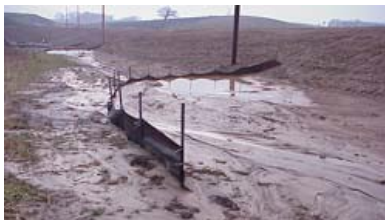
Figure 22. A silt fence full of sediment that needs maintenance.
