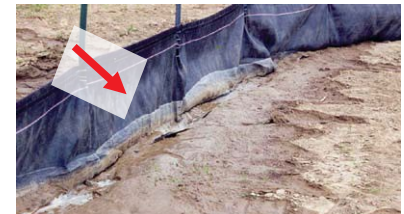
Figure 16. Poor compaction has resulted in infiltration and water flowing under this silt fence causing retained sediment washout.
