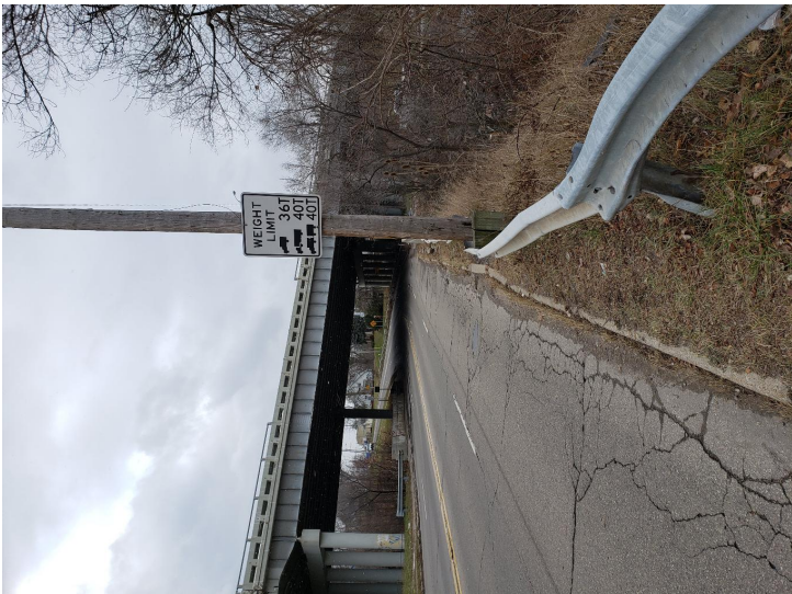
Document Name: 20181207_142745.jpg Category: Posting Span Number: Comments: Load Posting Sign 36/40/40 at Northwest quadrant
