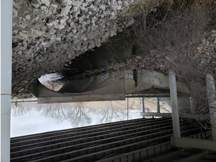
Document Name: 20181207_141037.jpg Category: Elevation Span Number: Comments: East Elevation looking west downstream
